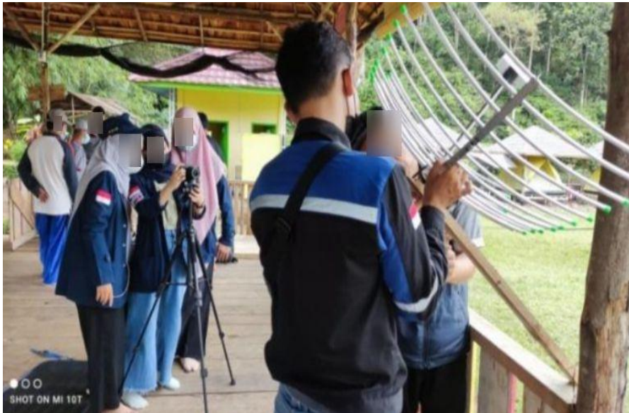
Figure 4. Installation of Cellphone and Internet Signal Booster Antenna Source: Adapted by the Author (2025) from UNIB Archives
